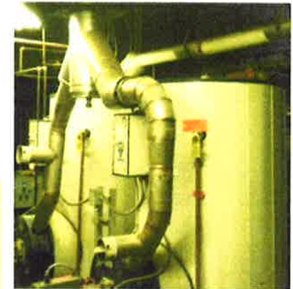
Domestic Hot Water Heaters
