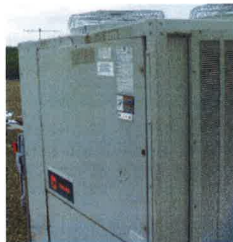
Condensing Unit on Roof
