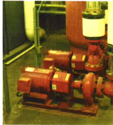
Hot Water Pumps
