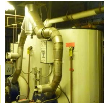
Domestic Hot Water Heaters
