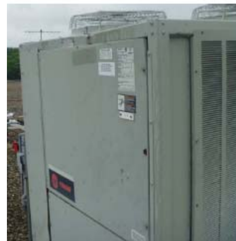
Condensing Unit on Roof
