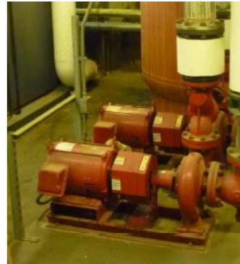
Hot Water Pumps
